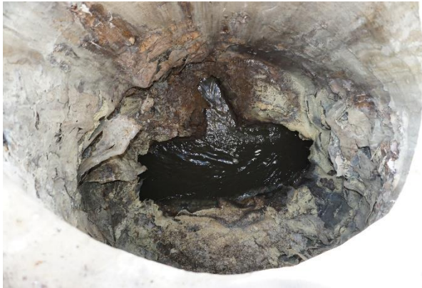
Failed Epoxy: Leaving concrete exposed
