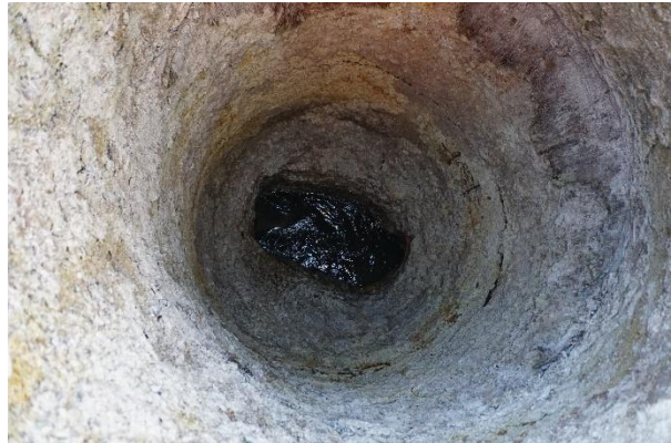
Exposed Rebar: Multiple sections
